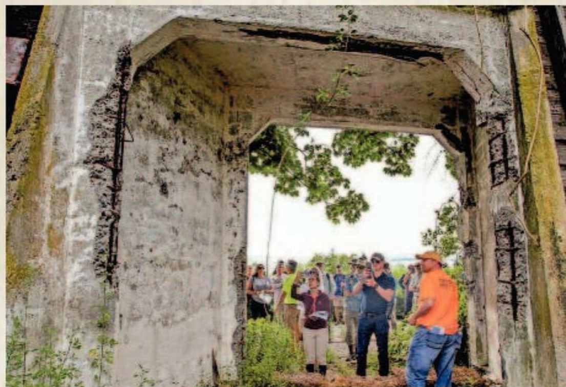
A bunker built to house torpedoes on Gould Island is explored by visitors on a 2019 tour. After World War II, torpedo operations were moved to another naval station on the West Coast, and the island fell into disuse. DAVID DELPOIO/THE PROVIDENCE JOURNAL
